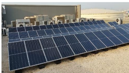
Fig. 1. Solar PV panels setup
