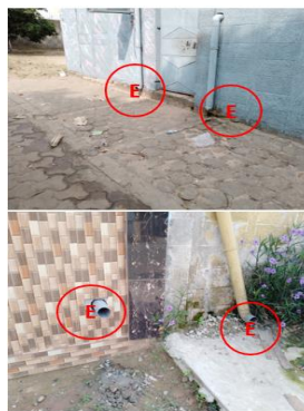
Plate 1: Gutters draining rainwater into the street
