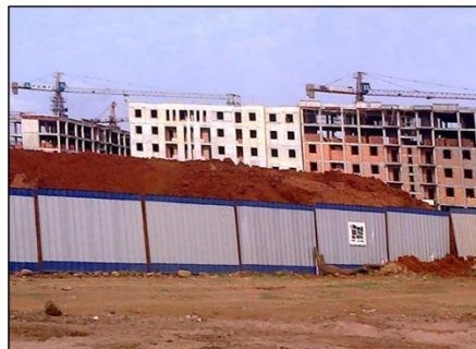
Figure: Landslide in Sidi Abdallah New City
