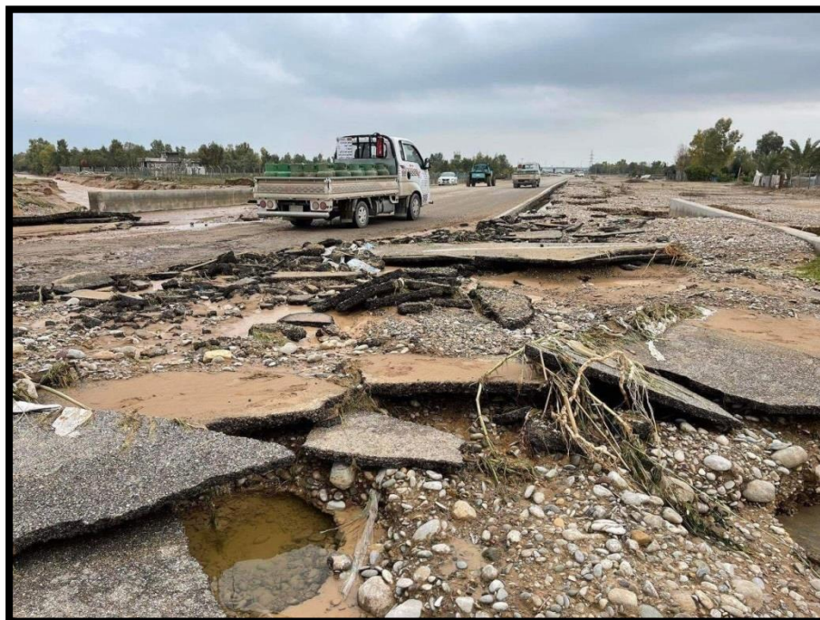
Figure 3: Road collapse due to floods in Kalar district
